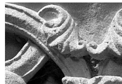
Senlis cathedral pier S9e(a)
